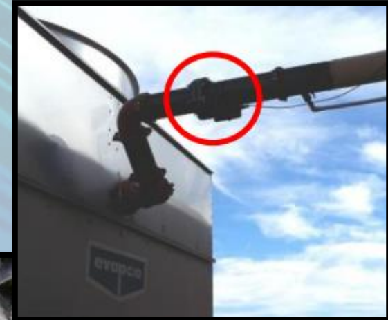
Installed HydroFLOW device.
