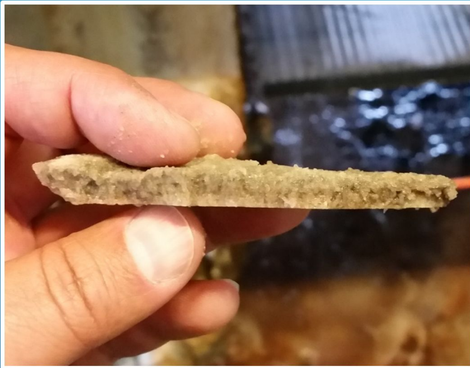
1/4 INCH STRUVITE BUILD-UP INSIDE THE BELT PRESS
