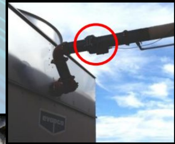
Installed HydroFLOW .device
